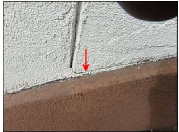
Delamination of EPS planton needs to be re-adhered prior to sealant joint application at planton perimeter; typical
