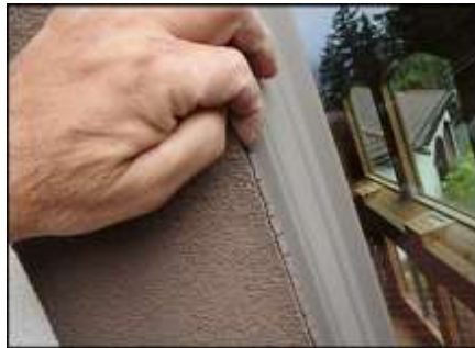
Sealant joint failure at window perimeter needs to be removed and replaced; typical
