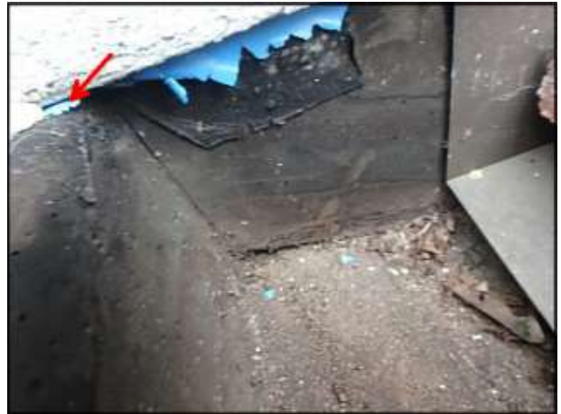
Torch down roofing to stucco needs sealant joint application; typical
