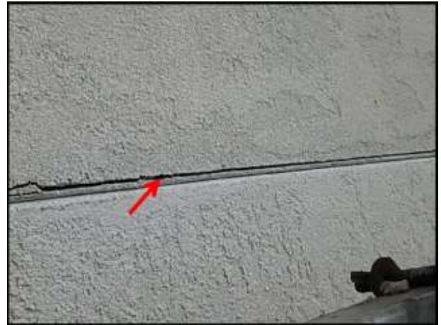
Crack at expansion joint needs to be sealed; typical
