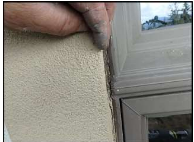
Sealant joint failure at window perimeter needs to be removed and replaced; typical
