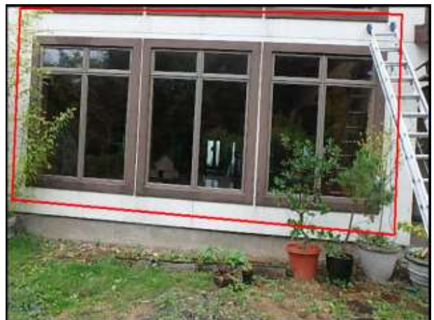
Approximate area of soft substrate at window perimeter needs to be removed and replaced (H5-I7)
