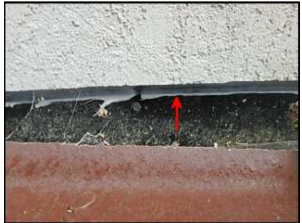
Roof flashing at stucco termination needs to be integrated into water-resistive barrier (H4-I4)
