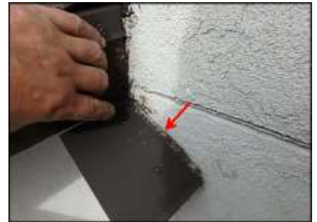
Roof and fascia terminations need sealant joint application; typical
