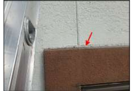
Delamination of EPS planton needs to be re-adhered prior to sealant joint application at planton perimeter; typical
