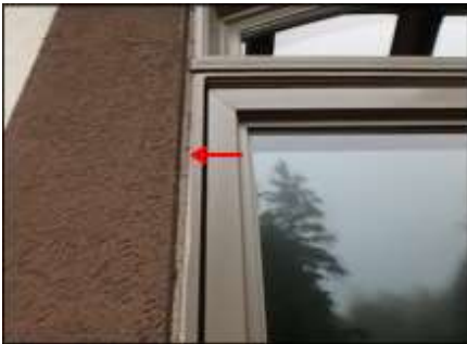
Sealant joint failure at window perimeter needs to be removed and replaced; typical
