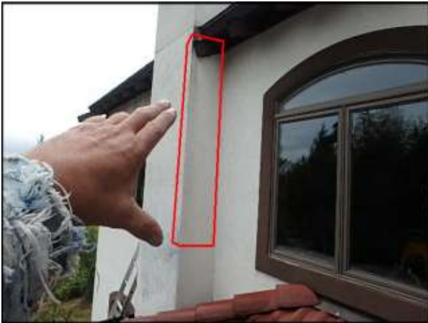
Approximate area of soft substrate below roof termination needs to be removed and replaced (E3-E4)
