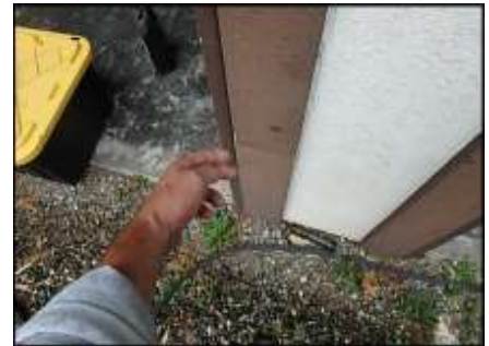
Recommend remediation of area of impact damage for aesthetic purposes (C7)
