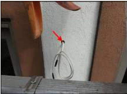
Penetration needs to be sealed; typical
