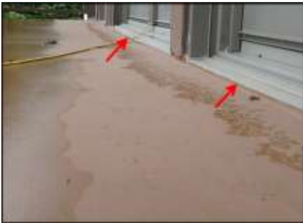
Deck doors need pan flashings installed; typical
