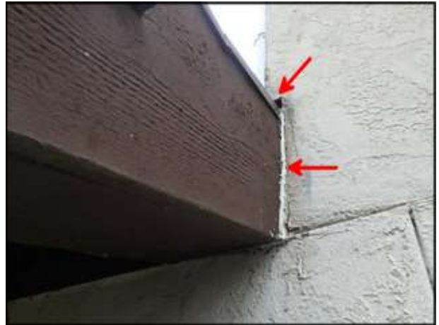
Roof and fascia terminations need sealant joint application; typical
