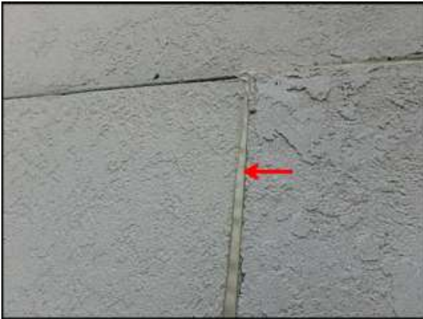
Aged sealant joint needs to be removed and replaced (D6)
