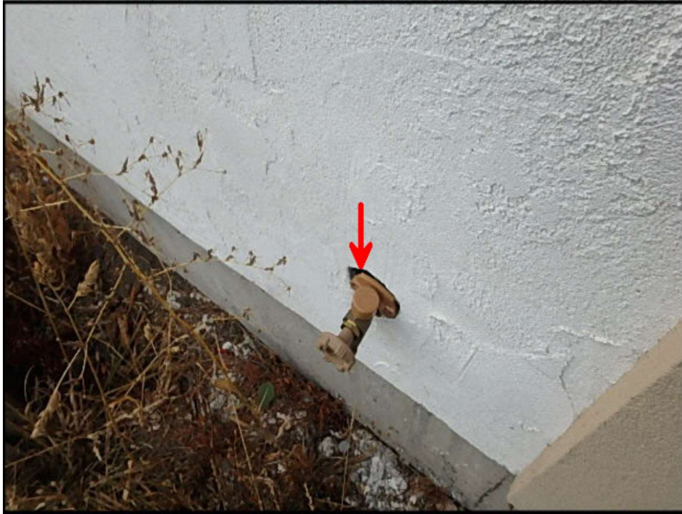
Hose bib penetration needs sealant joint application; typical
