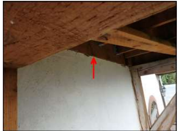
Deck ledger to stucco needs sealant joint application (E4-F4)
