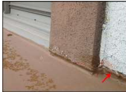
Deck to stucco needs flashing installed; typical
