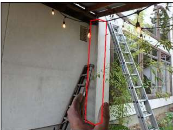
Approximate area of soft substrate below roof termination needs to be removed and replaced (H5-H7)
