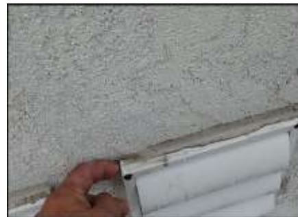
Sealant joint failure at vent penetration needs to be removed and replaced; typical
