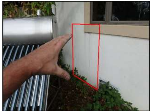
Approximate area of soft substrate below window needs to be removed and replaced (C7)
