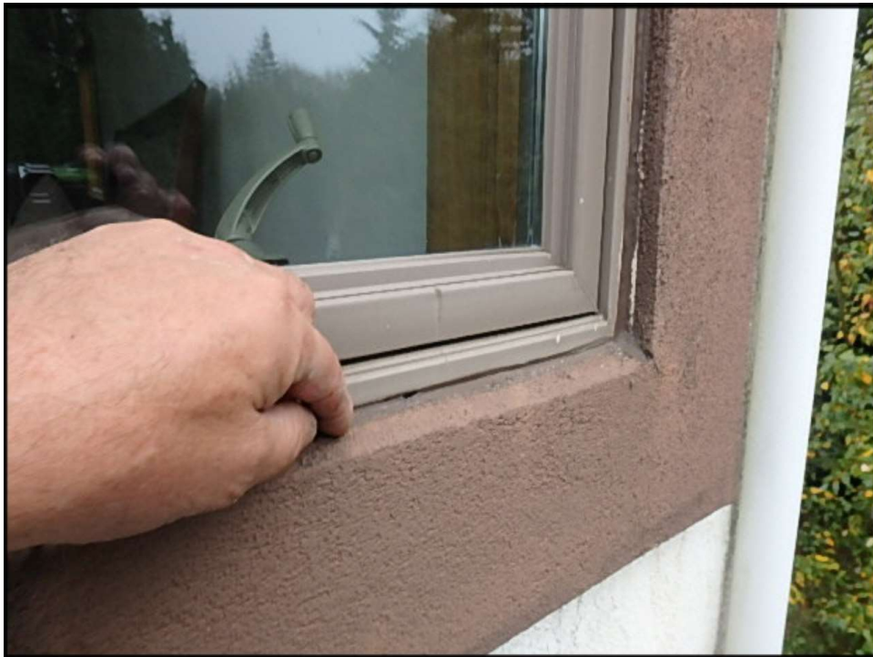
UV damaged sealant joint failing at window perimeter needs to be removed and replaced; typical
