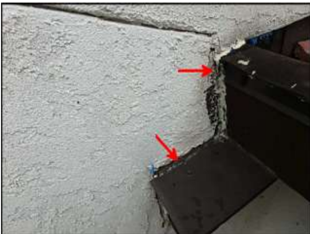
Fascia and beam terminations need sealant joint application; typical
