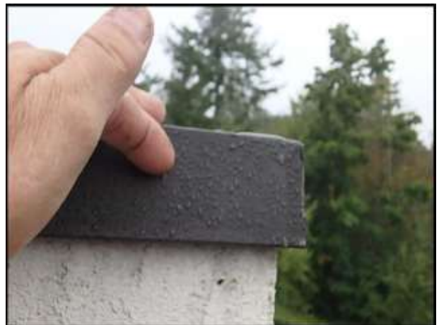
Chimney cap adequately extends over stucco to protect against moisture intrusion; typical
