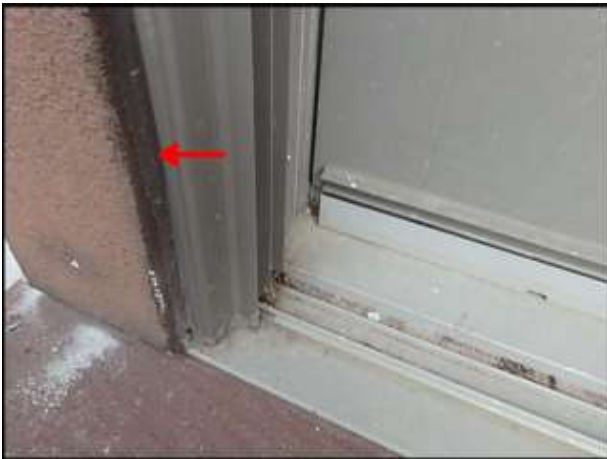
Sealant joint failure at door head and jambs needs to be removed and replaced; typical
