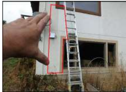
Approximate area of soft substrate at windows needs to be removed and replaced (C5-D7)
