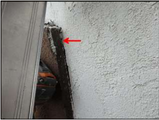
Delamination of EPS planton needs to be re-adhered prior to sealant joint application at planton perimeter; typical
