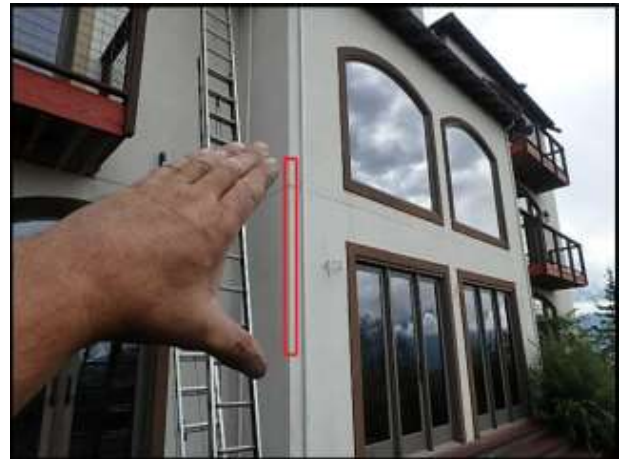
Approximate area of soft substrate at corner needs to be removed and replaced (D6)
