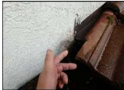
Torch down adequately extends behind stucco to protect against moisture intrusion at cut & turned kickout flashing installed at roof termination; typical
