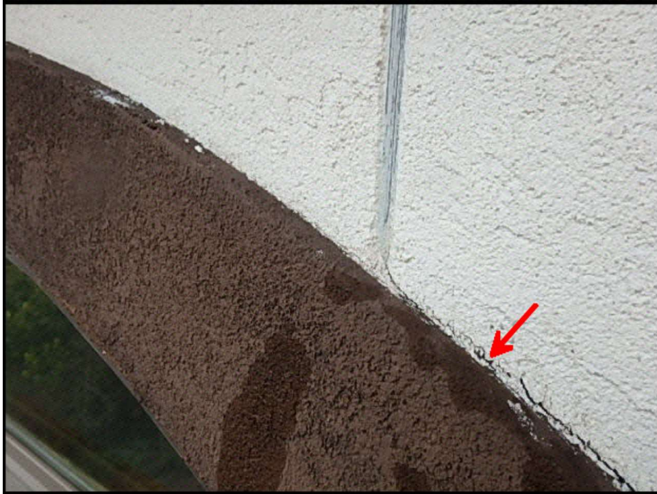
Delamination of EPS planton needs to be re-adhered prior to sealant joint application at planton perimeter; typical
