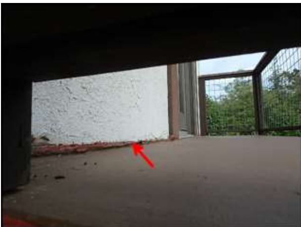
Deck to stucco needs flashing installed; typical
