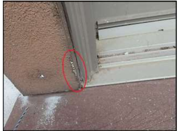
Area of impact damage needs remediation (D6)
