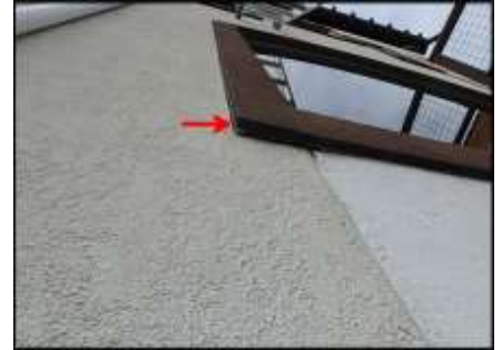
Delamination of EPS planton needs to be re-adhered prior to sealant joint application at planton perimeter; typical
