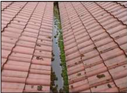
Roof valley needs to be cleared of debris to allow for unobstructed water flow; typical
