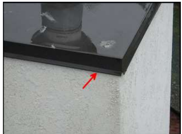
Chimney cap adequately extends over stucco to protect against moisture intrusion; typical
