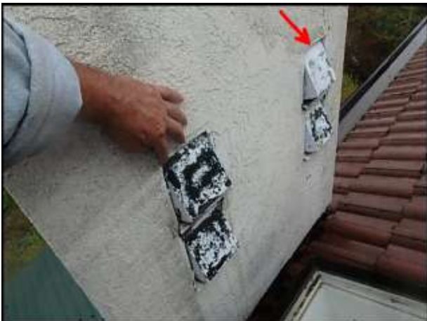
Vent penetrations need sealant joint application (E2)
