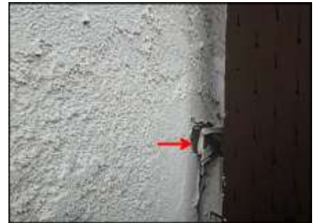
Deck terminations need end dam flashings installed (E4, F4)
