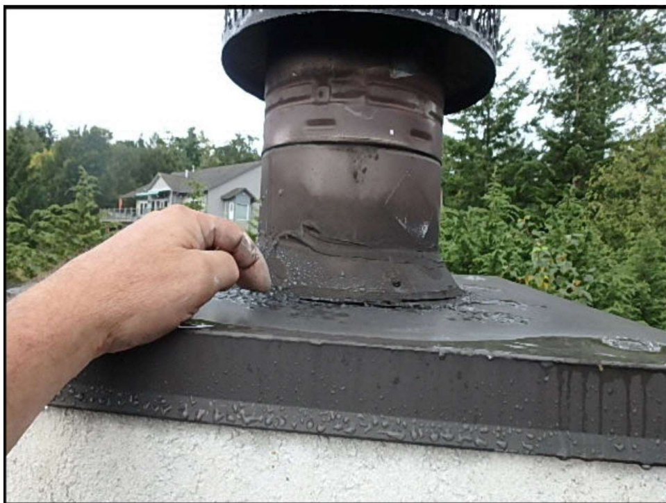
Chimney cap adequately extends over stucco to protect against moisture intrusion; typical
