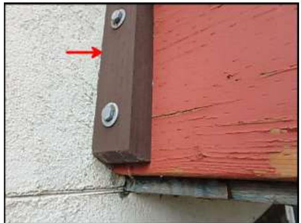
Deck termination needs sealant joint application; typical
