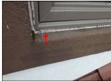
Sealant joint failure at window perimeter needs to be removed and replaced; typical
