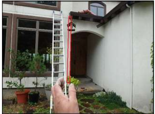
Approximate area of soft substrate below roof termination needs to be removed and replaced (I5-J7)
