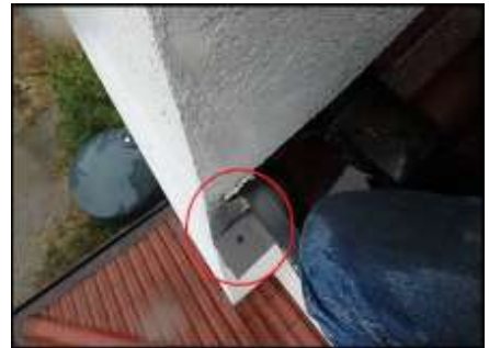
Roof termination needs further evaluation to determine necessary remediation upon remediation of soft substrate below (E3)
