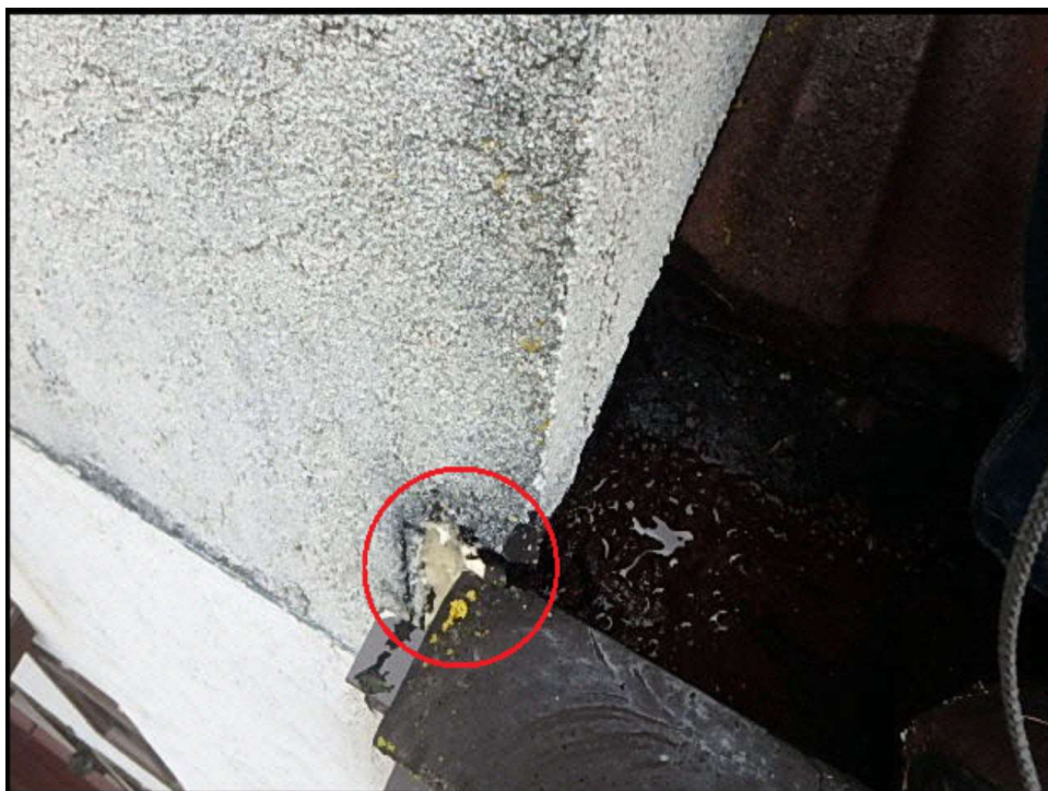
Roof termination needs sealant joint application; typical
