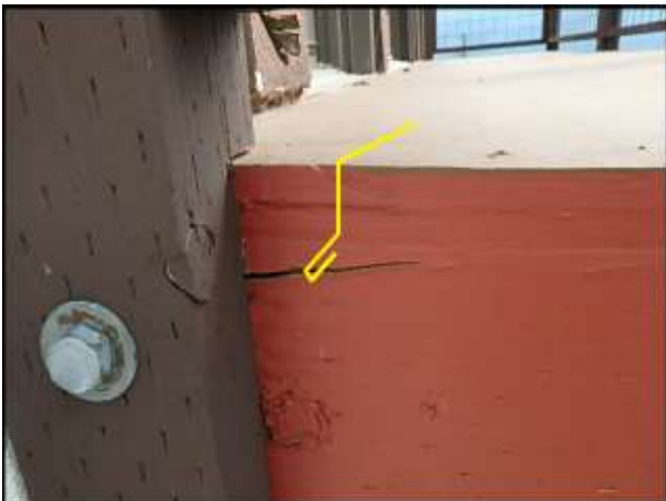
Deck to fascia needs drip flashing installed; typical
