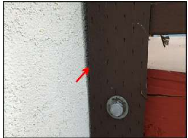
Deck termination needs end dam flashing installed; typical
