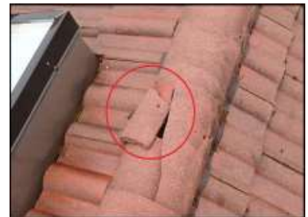
Broken roof tile needs to be replaced; typical
