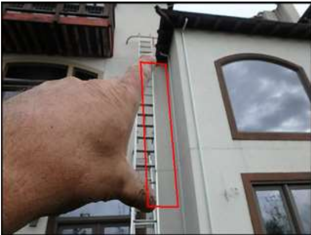
Approximate area of soft substrate below roof termination needs to be removed and replaced (D5-D6)
