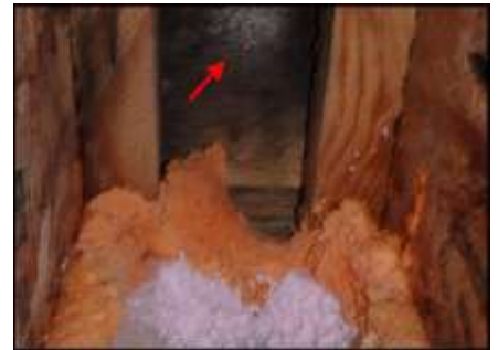
Visible water damaged plywood sheathing at deck needs to be removed and replaced; typical
