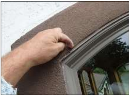
Sealant joint failure at window perimeter needs to be removed and replaced; typical
