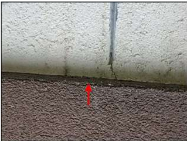
Delamination of EPS planton needs to be re-adhered prior to sealant joint application at planton perimeter; typical
