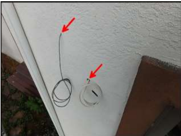
Penetrations need to be sealed; typical
