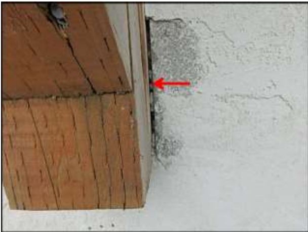
Deck supports need sealant joint application (E4, F4)
