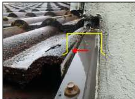
Flashing at roof termination needs counter cap flashing installed; typical
