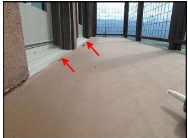
Deck doors need pan flashings installed; typical
