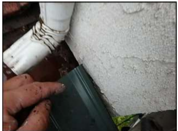
Roof termination needs flashing installation upon remediation of soft substrate below (H5)
