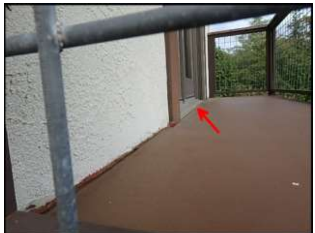
Deck door needs pan flashings installed; typical
