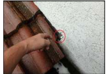
Torch down adequately extends behind stucco to protect against moisture intrusion at cut & turned kickout flashing installed at roof termination; typical
