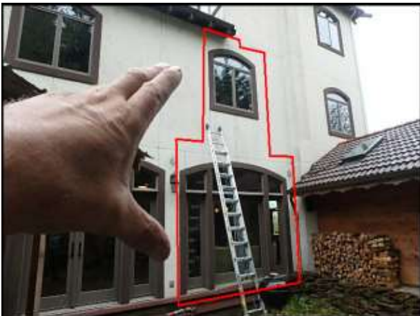
Approximate area of soft substrate below roof termination needs to be removed and replaced (G2-H6)
