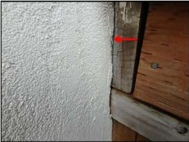
Deck fascia termination needs sealant joint application (E4, F4)
