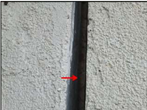
Visible oriented strand board at joint; joint needs sealant joint installed (D6)
