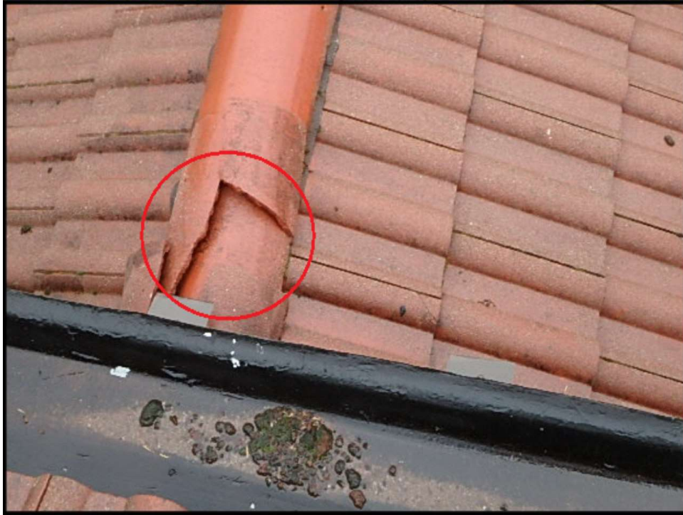
Broken roof tile needs to be replaced; typical
