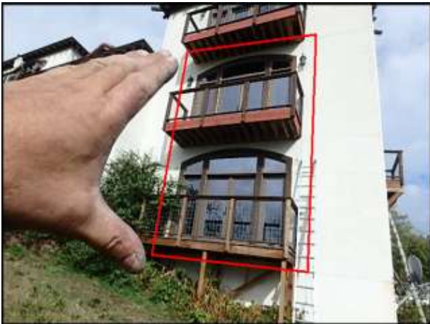
Approximate area of soft substrate at decks needs to be removed and replaced (E3-G7)
