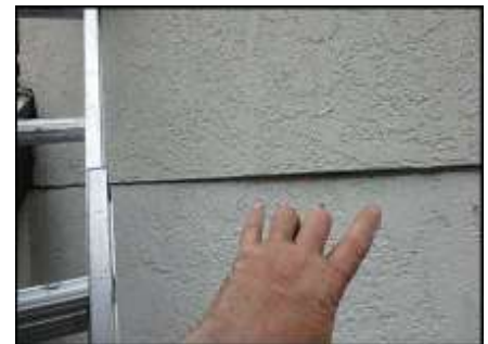
Deflection observed at floor line appears to be due to stucco installation over earthquake strap (D4)
