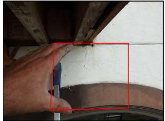
Approximate area of soft substrate below deck needs to be removed and replaced (D6)
