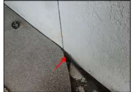
No remediation necessary at concrete poured to base of stucco at entry due installation of rubber flashing to protect against moisture intrusion (A6)
