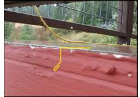
Deck to fascia needs drip flashing installed; typical
