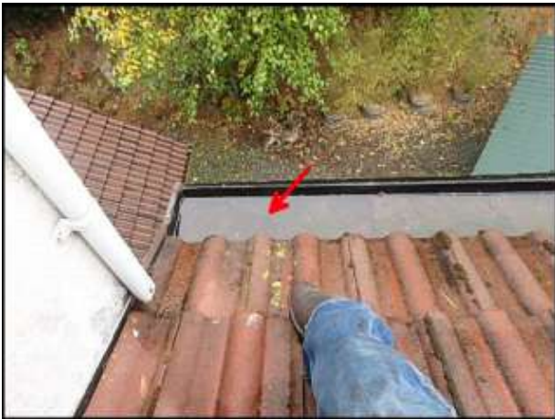
Gutter needs to be re-sloped upon remediation of soft substrate below to allow for unobstructed water flow (E2-G2)
