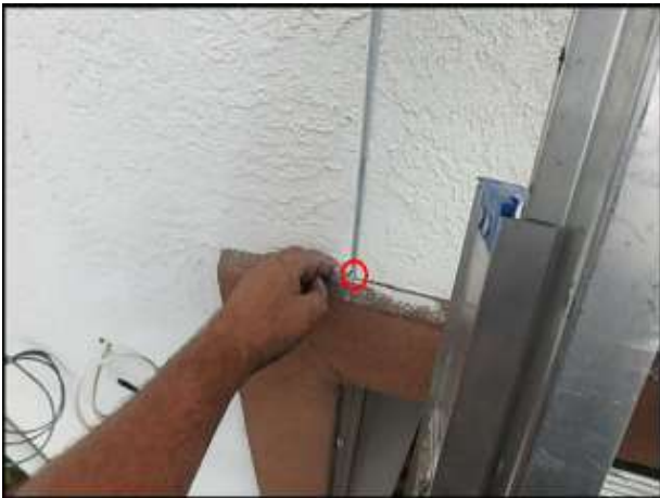
Control joint termination needs to be sealed; typical
