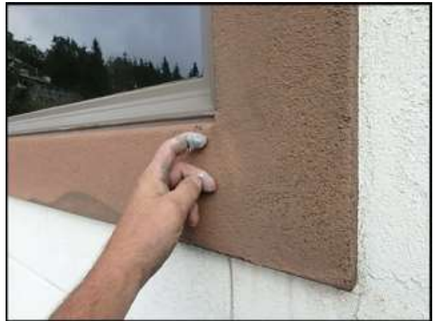
Hairline crack at EPS planton needs elastomeric coating application; typical
